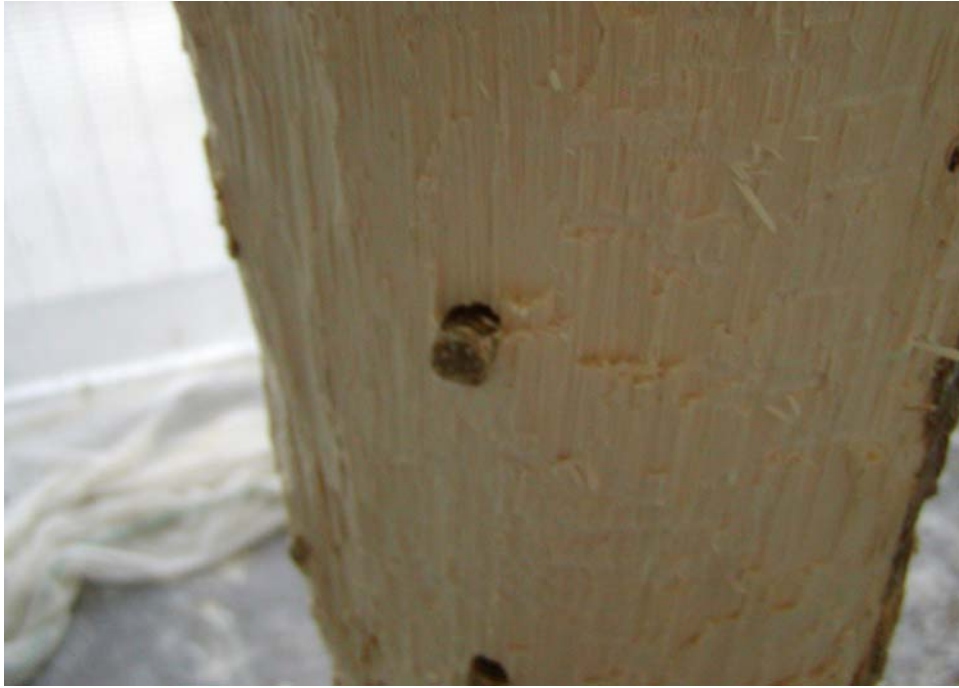
Figure 5: Plug treatment with signs of extensive amounts of pole damage surrounding the plug. Plug showed no effect on reducing the amount of wood removed from untreated surfaces adjacent to the plugs.
