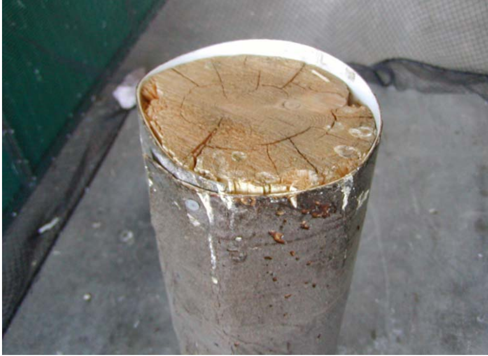
Figure 3: IStop-CC™ Epoxy Resin System, wrap treatment. A precured sheet of epoxy and PVC sheeting was nailed to the pole and cut to fit. Top of pole, as seen, was left exposed.
